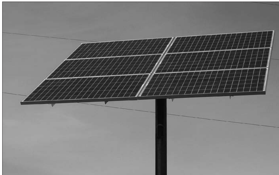
A solar panel installed at Patrick's home in Goldendale catches sunlight.
