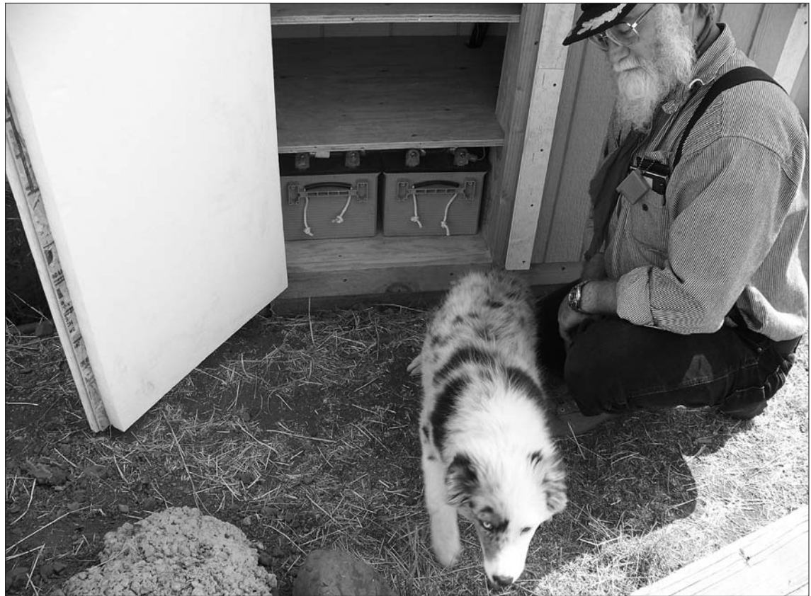
KPUD customer Patrick Cramer and his Australian shepherd, Catch, show off the direct-current output from the solar cells that is stored in batteries.
